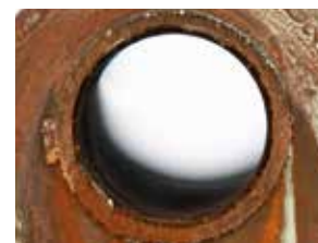
Tankless with X3 Technology: Still running after 19.7 years of operation and 460,000 gallons
