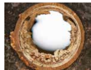
Unprotected tankless: Failed at 5.8 years of operation and 136,000 gallons
