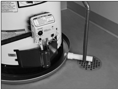
Figure 23 - Metal drain pan piped to drain.
